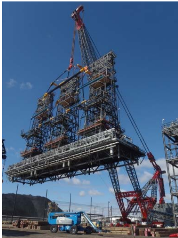
Figure 7: ALE completed a series of record-breaking lifts at an oil refinery in Texas, USA. The crane's variable ballast radius makes it possible to perform lifts at a 54 metre outreach from a single position, eliminating cost-intensive dismantling and repositioning.
